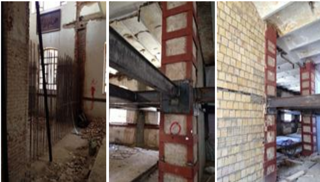
Fig. 9. Renovation of Tabriz Islamic Art University library, reinforcing brick columns with metal and concrete elements.
