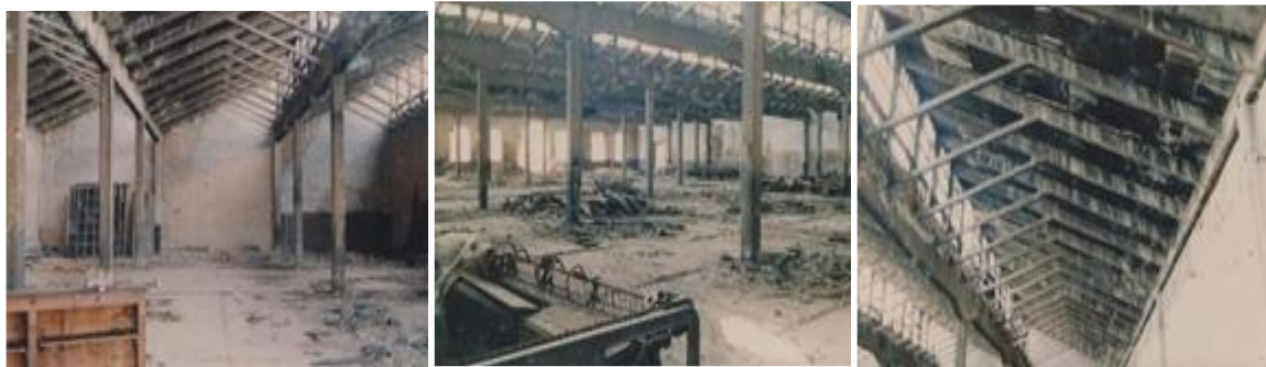
Fig. 6. The Pashmina building before renovation, the structural system, and the precision of execution were the aesthetic and identity characteristics of the work.
